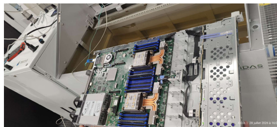
Cisco server ready for immersion
